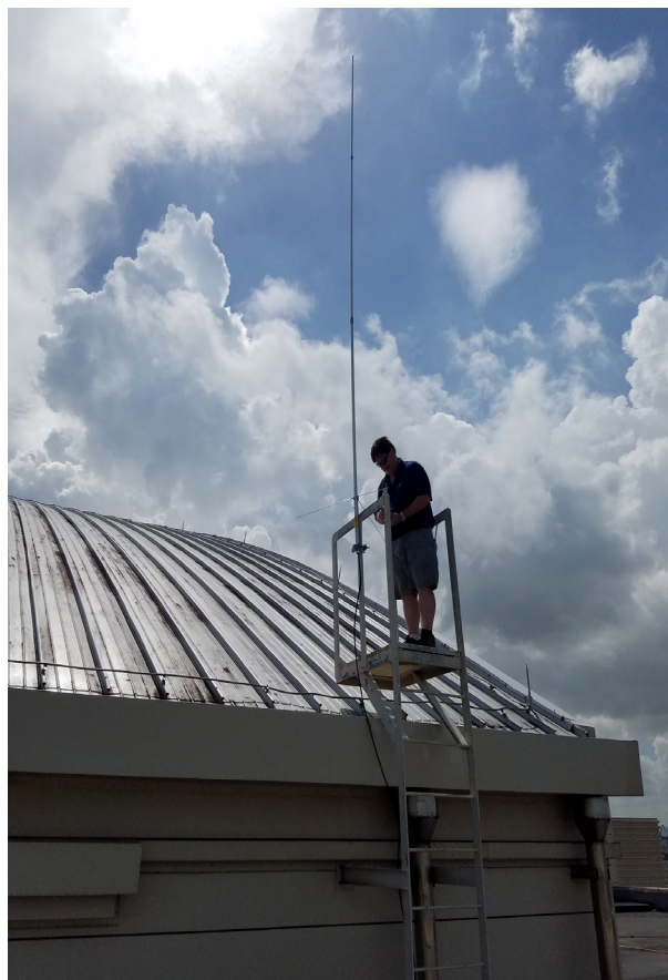
Volunteer Gary Sessums, KC5QCN, installs a VHF antenna on the roof of the Puerto Rico Convention Center. [Mike Corey, KI1U, photo]
