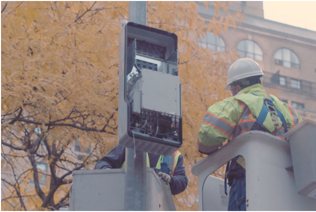
A crew works with AT&T to install a small cell antenna in New York City. Photo: Thomas Di Fonzo for the Wall Street Journal
